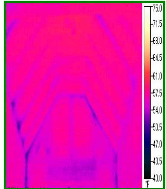
Thermal Infrared Image (East Dormer shows no exception)
